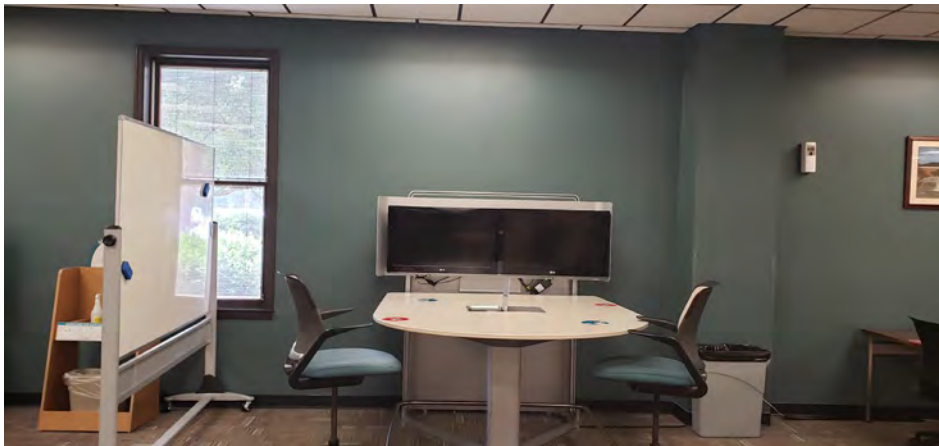
Drywall/joint compound located on the front wall of the 1st & 2nd floors
