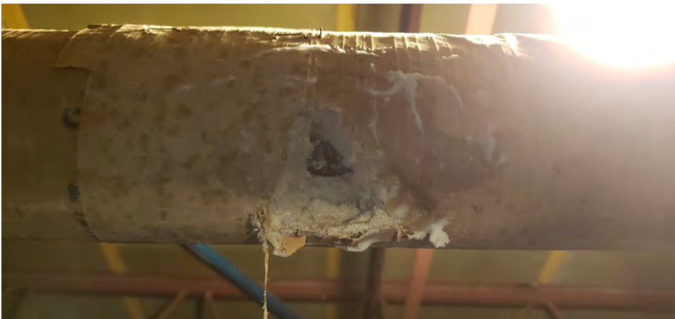
Pipe insulation on hard small (approximately 6") pipes - located in the 2nd floor mechanical room (white inner insulation)
