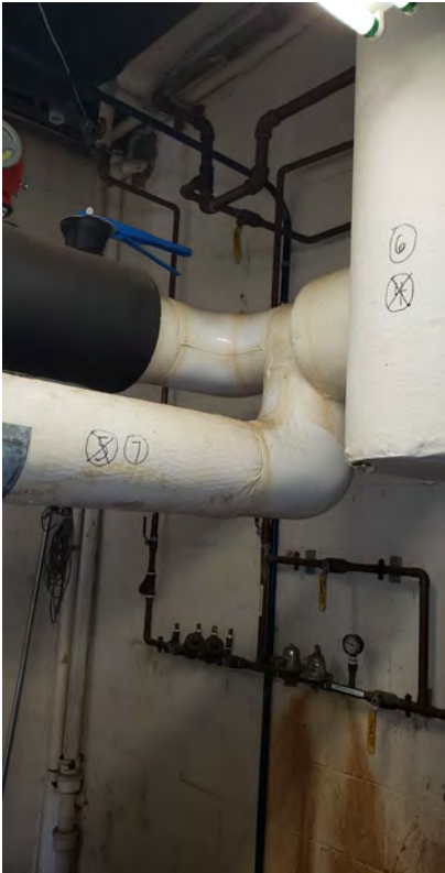
Insulation covering on approximately 6-inch fiberglass insulated pipe connected to the "Chiller" tank located in the front left mechanical room
