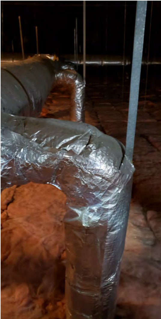
Duct tape on HVAC equipment - located in the 2nd floor mechanical rooms, etc.
