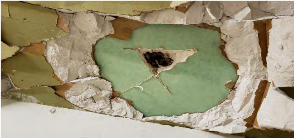
Green ceiling board system - located in the 2nd floor mechanical room, etc.
