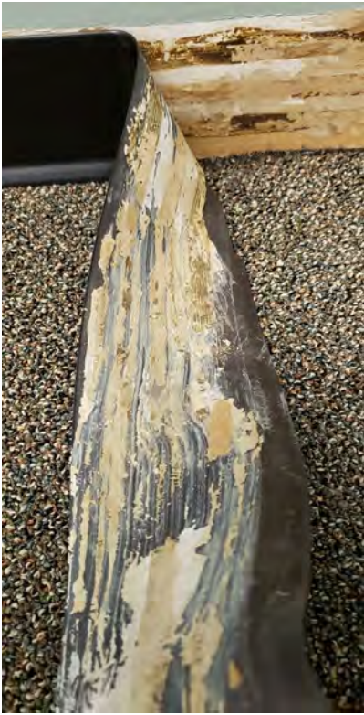
Mastic associated with base cove installed with brown carpet located in the rear left area of the 2nd floor
