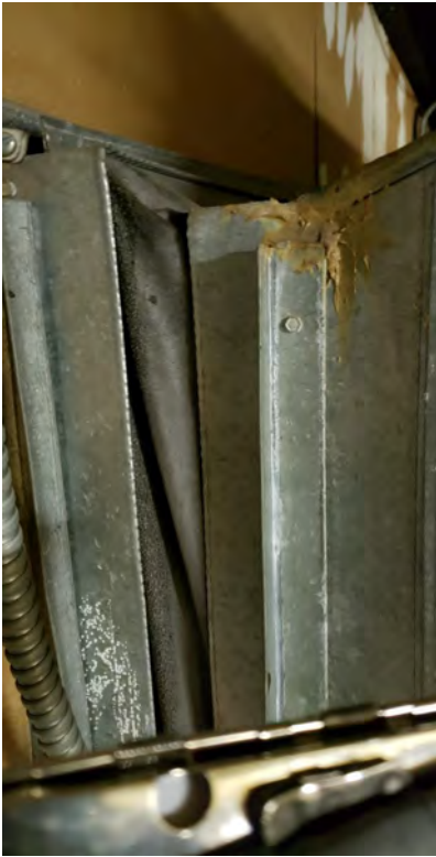
Expansion joint and mastic on HVAC equipment - located in the 1st and 2nd floor mechanical rooms, etc. Tan mastic tested positive for asbestos
