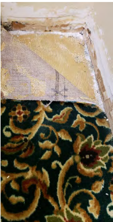
Mastic associated with green flower patterned carpet located in the front right area of the 2nd floor
