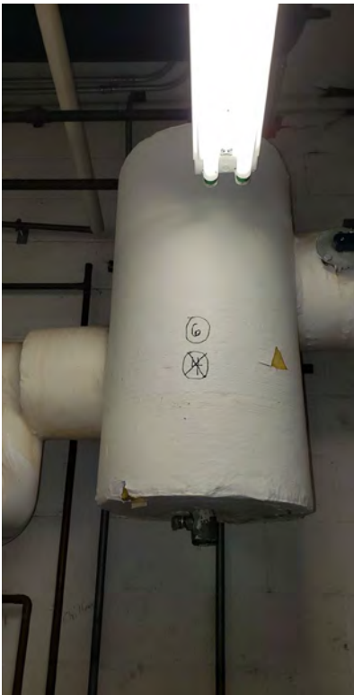
Insulation covering on "Chiller" tank located in the front left mechanical room
