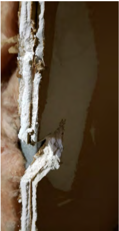
Dyrwall/joint compound (two layers in some areas) - located in the 1st and 2nd floor mechanical rooms, etc.
