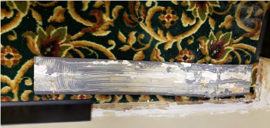
Mastic associated with base cove installed with green flower patterned carpet located in the front right area of the 2nd floor
