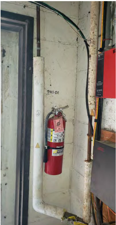
Insulation covering on approximately 3-inch fiberglass insulated pipe connected to the city water pipe located in the front left mechanical room
