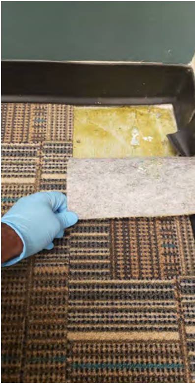
Mastic associated with multicolored carpet located throughout the 1st & 2nd floors
