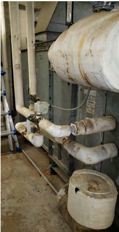
Insulation covering on approximately 2-inch fiberglass insulated pipe connected to the air handler located in the front left mechanical room
