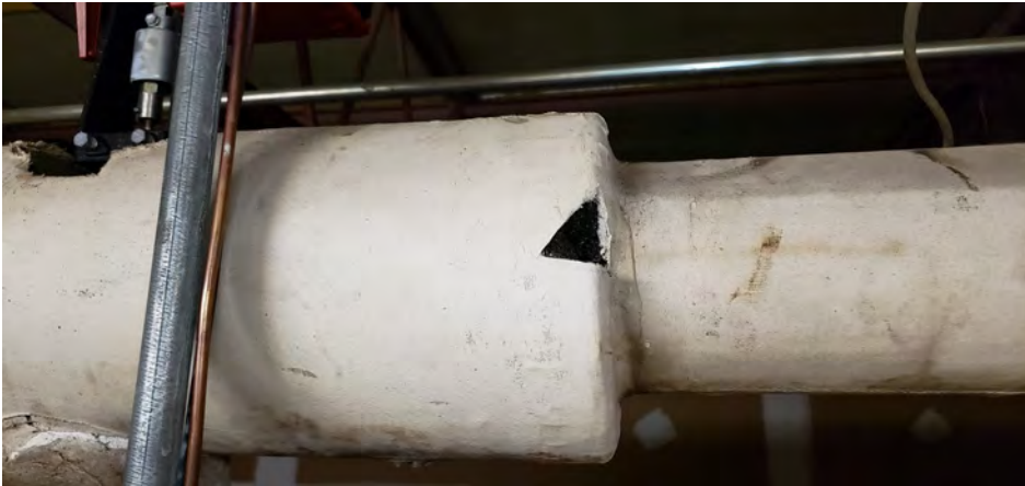
Flange insulation on hard large (approximately 18") pipes - located in the 1st and 2nd floor mechanical rooms
