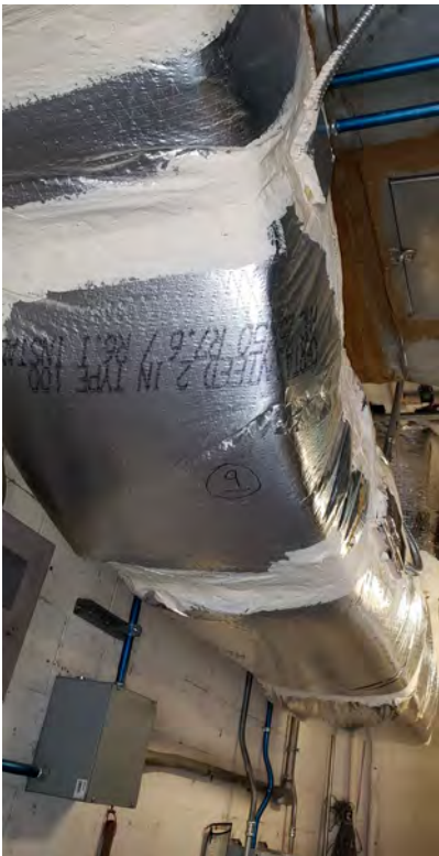
White mastic on HVAC ductwork located in the front left mechanical room
