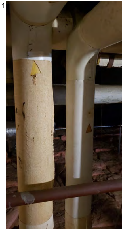
Pipe insulation covering on large (approximately 18") soft/fiberglass insulated pipes located in the 1st and 2nd floor mechanical rooms
