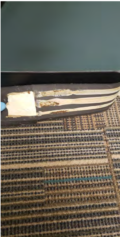
Mastic associated with base cove installed with multicolored carpet located throughout the 1st & 2nd floors
