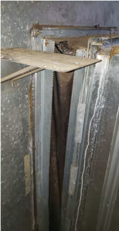
HVAC system expansion joint located in the front left mechanical room
