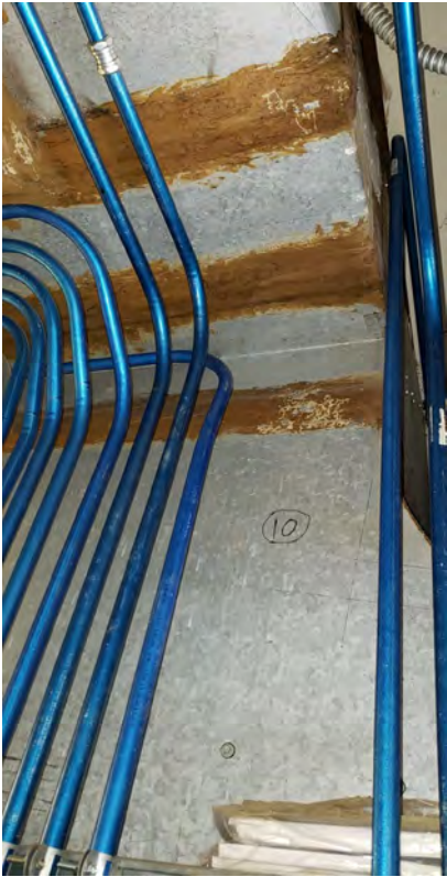
Brown mastic on HVAC ductwork located in the front left mechanical room
