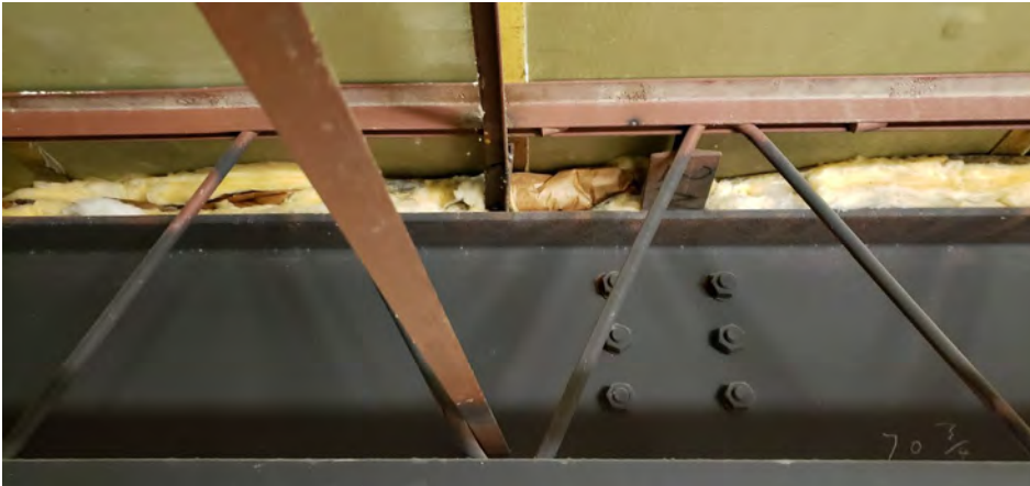
Batt insulation paper backing - located in the 1st and 2nd floor mechanical rooms, etc.
