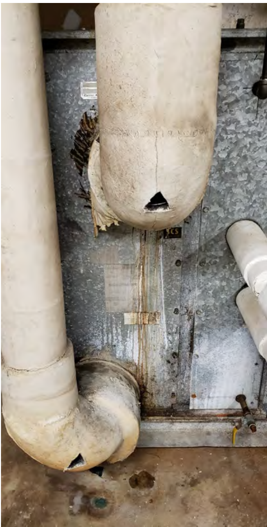
Elbow insulation on hard large (approximately 18") pipes - located in the 1st and 2nd floor mechanical rooms
