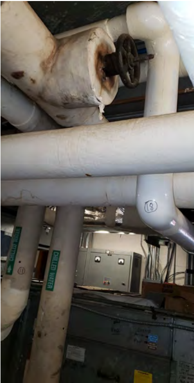
Insulation on approximately 4-inch hard insulated pipe connected to the chilled water line located in the front left mechanical room
