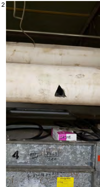
Pipe insulation on large (approximately 18") hard pipes - located in the 1st and 2nd floor mechanical rooms (black inner insulation)
