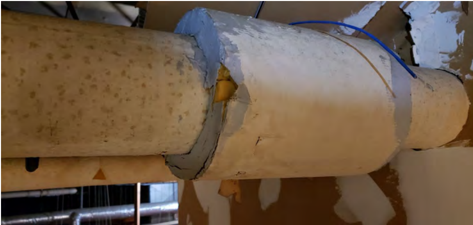
Flange covering on large (approximately 18") soft pipes - located in the 1st and 2nd floor mechanical rooms
