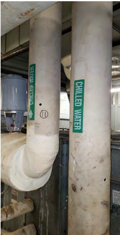
Insulation on approximately 6-inch Chilled water pipe located in the front left mechanical room
