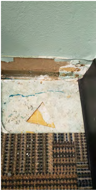
Vinyl flooring system under carpet in office areas on the 1st floor Two layers in some areas
