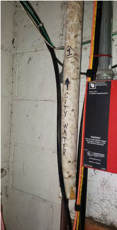
Insulation covering on approximately 2-inch fiberglass insulated city water pipe located in the front left mechanical room
