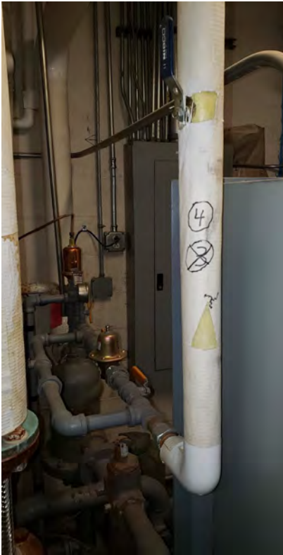
Insulation covering on approximately 2-inch fiberglass insulated hot water make-up pipe located in the front left mechanical room
