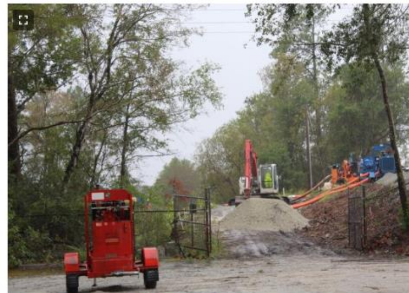
Santee Cooper crews have been working all week hoping to prevent ash from two ash ponds at the old Grainger Sta Plant from seeping into the Waccamaw River.
